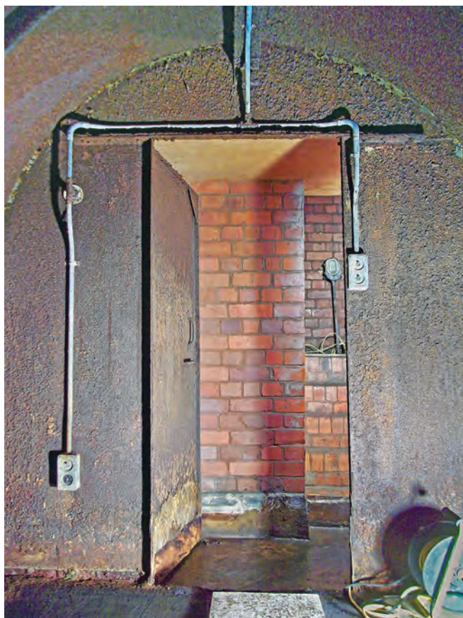
Looking out of the first shelter, the gas-proof door is seen and, to the right, steps up to the upper landing. Note the metal conduit for power cables. To the left of the door a 5A 3-pin power socket and switch is seen with two light switches to the right of the door. A Wigan bulkhead light is seen on the upper landing.
